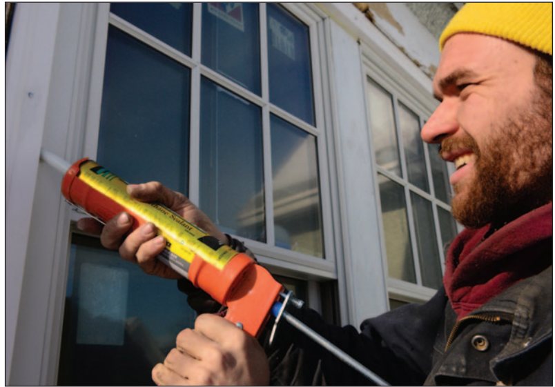
The average American family spends $2,000 annually on energy bills. Unfortunately, much of that money is wasted through air leaks in the home. Applying caulk around windows, doors, electrical wiring and plumbing can save energy and money. Photo credit: Rare Form Properties
