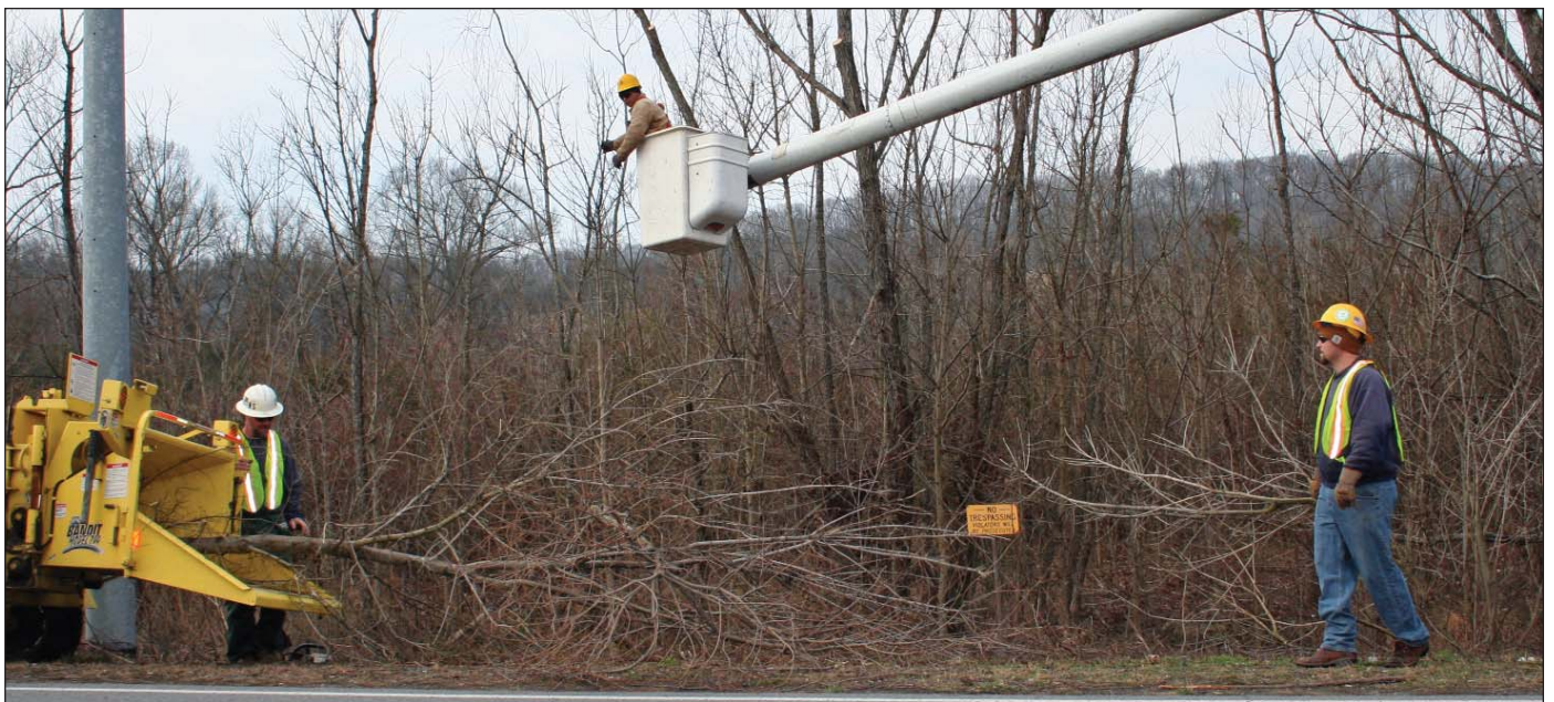
A three-man crew from Wolf Tree Experts works to clear the right-of-way along the Tennessee Waltz Parkway in Ashland City. From left are Nick Simpson, foreman, Felix Salamanca (in bucket) and Anthony Clark.
