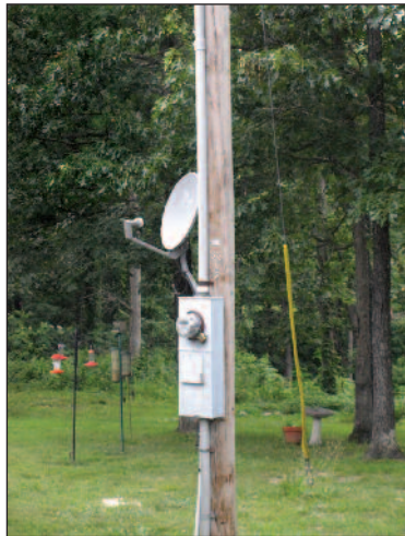
Satellite dishes and other unauthorized attachments must be removed to protect lineworkers. Source: Crawford Electric Cooperative
