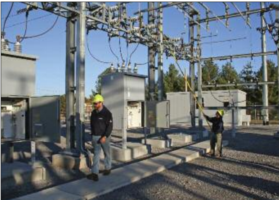
Substation technicians Ricky Cooksey, left, and Danny Smith work to restore power after an outage by switching the electrical load from one substation breaker to another.
